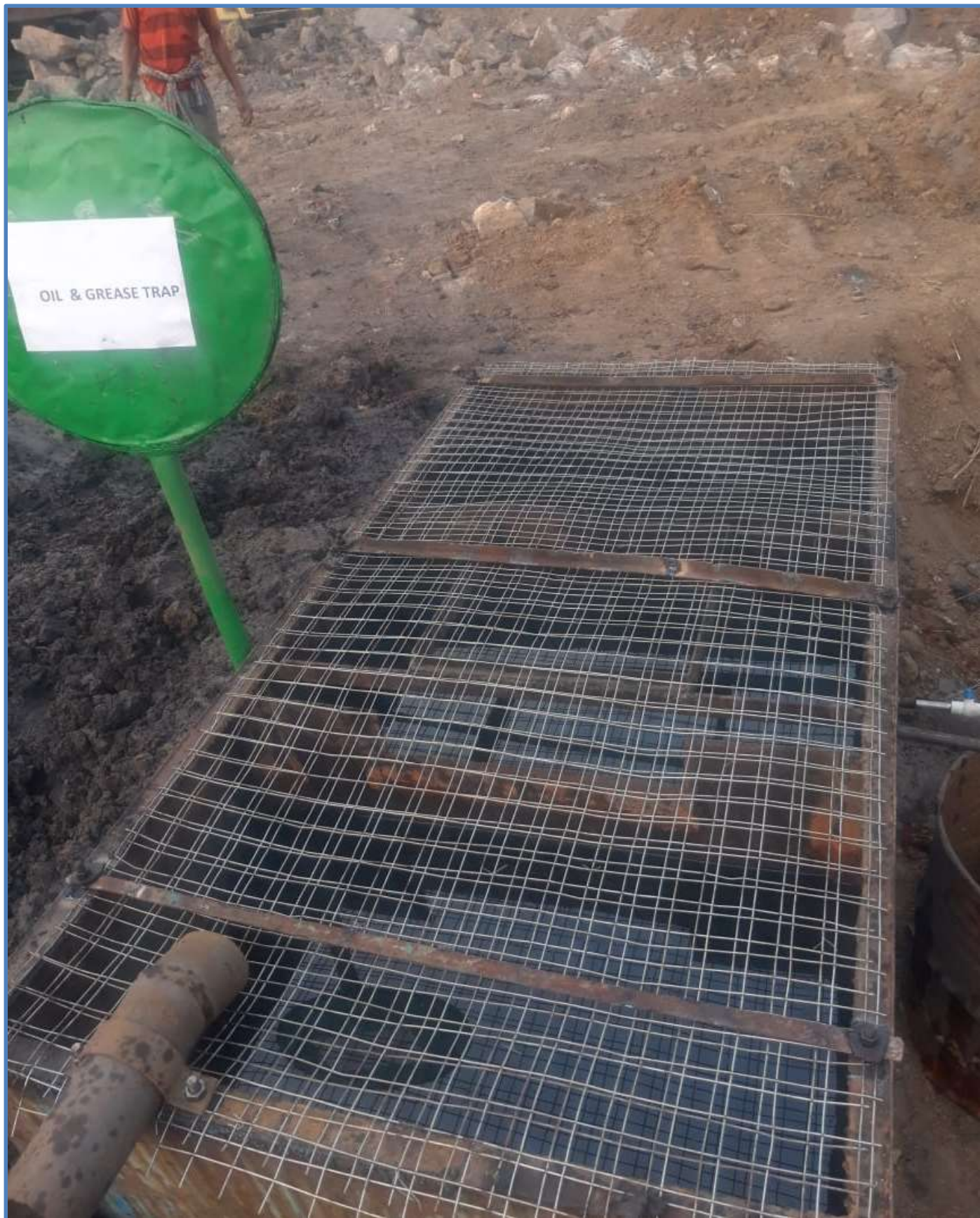
Picture 5 – Oil & Grease Trap
